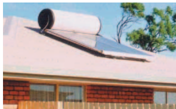
Domestic solar hot water unit Photo: Energy SA
