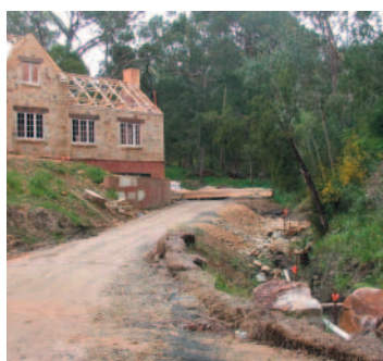
Housing constructed 3 metres from a watercourse Photo: P. Hazell, EPA
