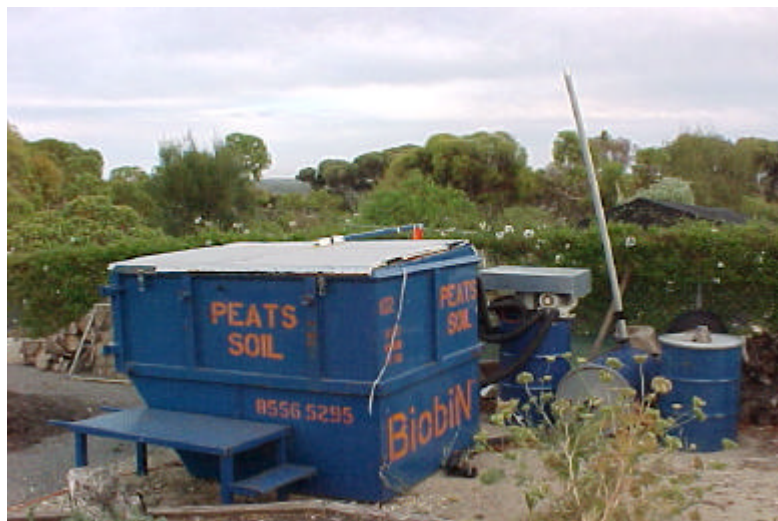
Figure 2: BiobiN™ showing pump and aeration system + biofilter stack (trial 2)
