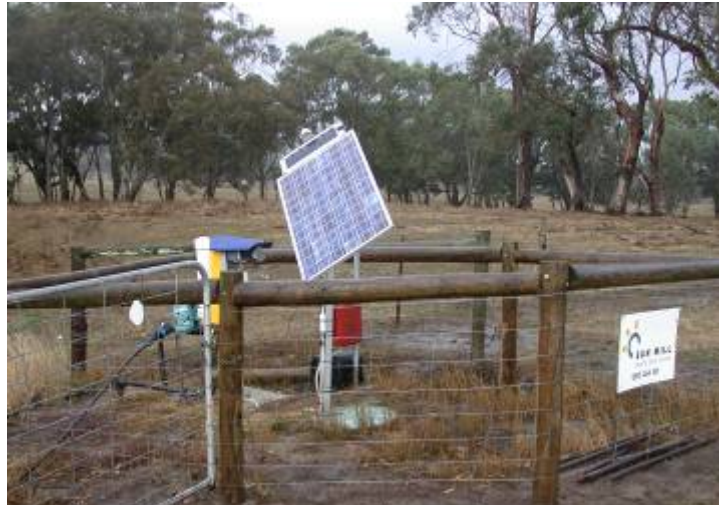
Plate 5 This solar pump was installed by the landholder as part of the off-stream watering system
